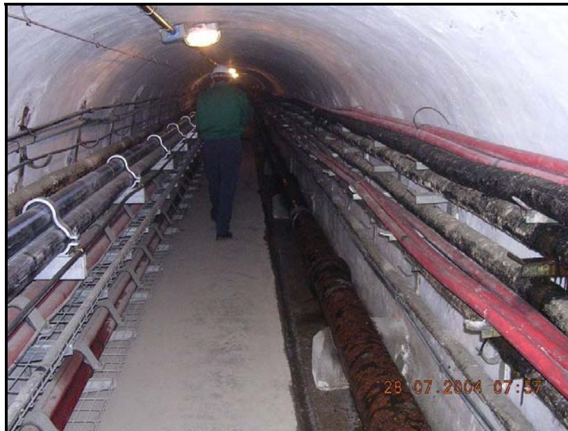
Figure 11 -- Buried Utilidor System
