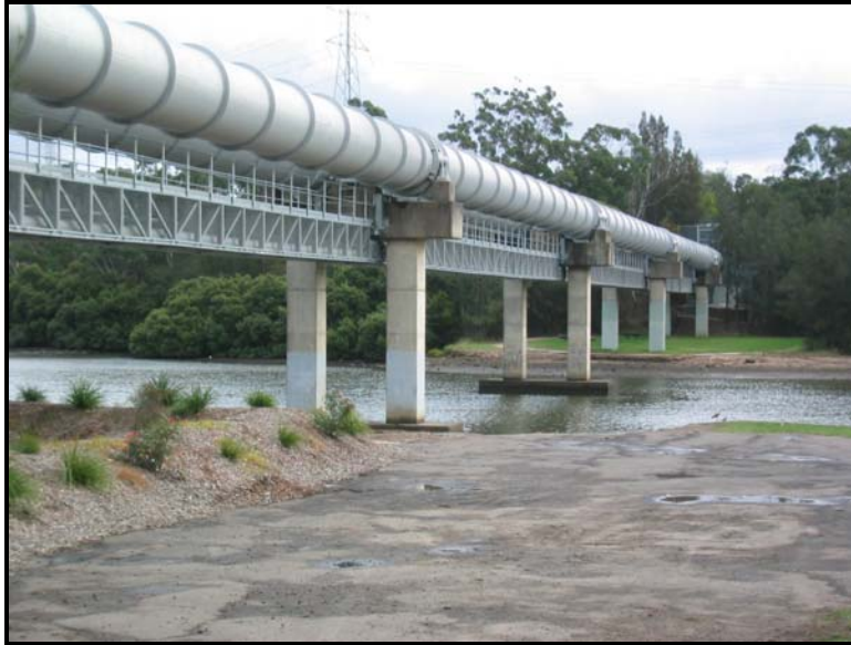
Figure 12 -- Above Ground Utilidor System
