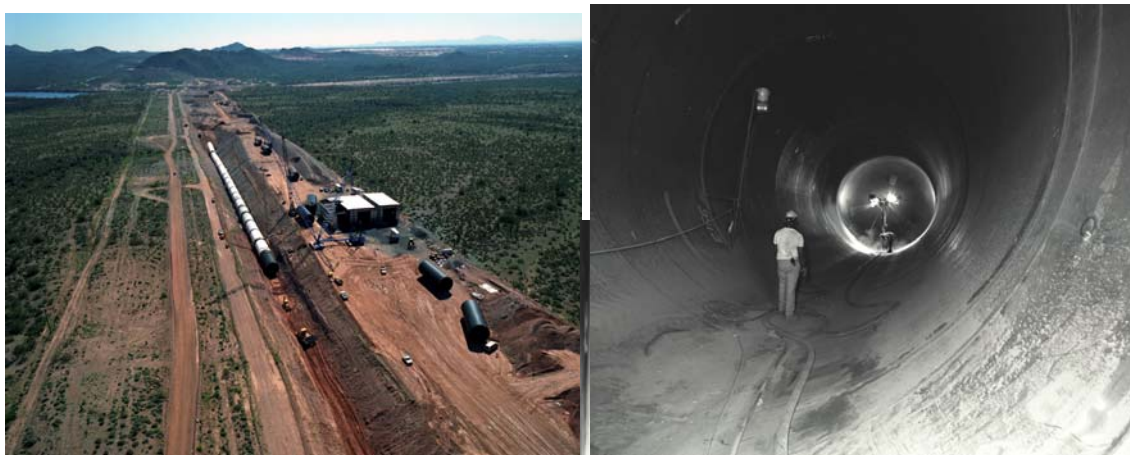
Figure 24 Construction of the large “tunnel” (inverted siphon) in the Colorado River Aqueduct.
